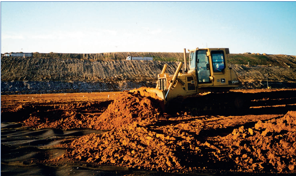
Sarasota, FL, landfill, Tendrain for leachate collection. Kent County, MI, Tendrain strips for leachate collection. Waverly, VA, landfill, Tendrain for leakage detection.
